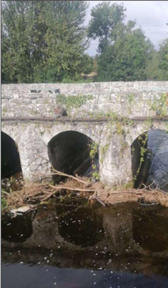
Plate 6 Debris at base of Dunkellin Bridge
